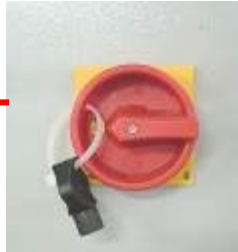
MAINS SUPPLY ISOLATOR
