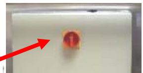
PROVER MAIN ISOLATOR
